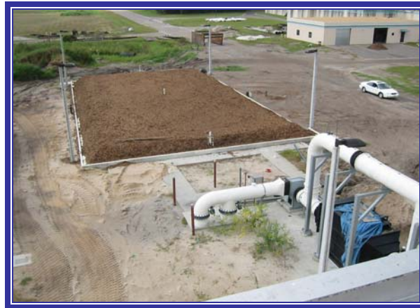
Wood Chip Biofilter
