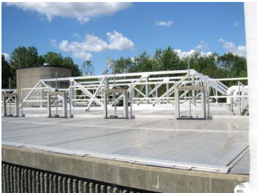
Aluminum covers on the grit tanks at the WCWTP
