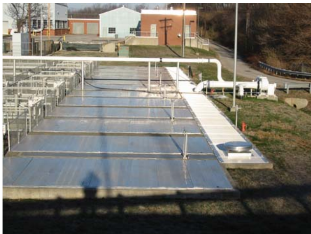
Primary Effluent Weir and Channel Covers
