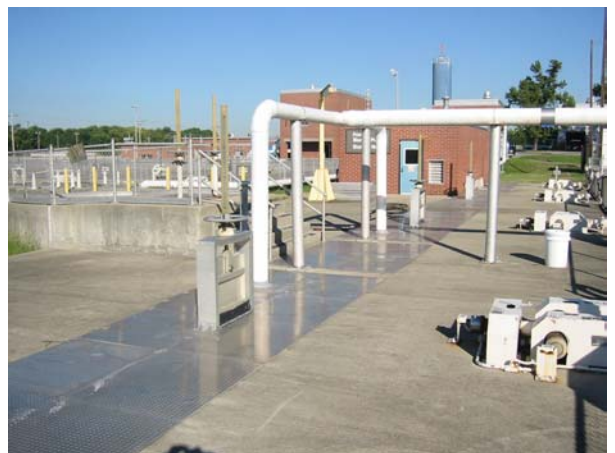
Primary Influent Channel Covers and FRP Duct
