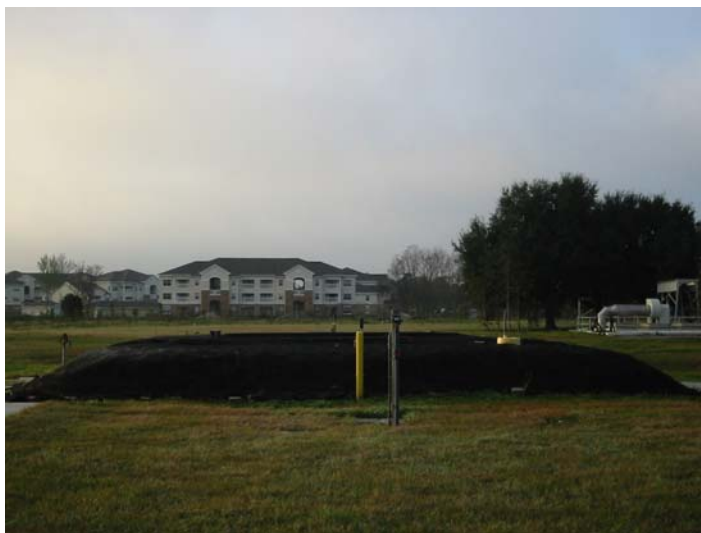
In-Ground Biofilter with Wood Chip Media
