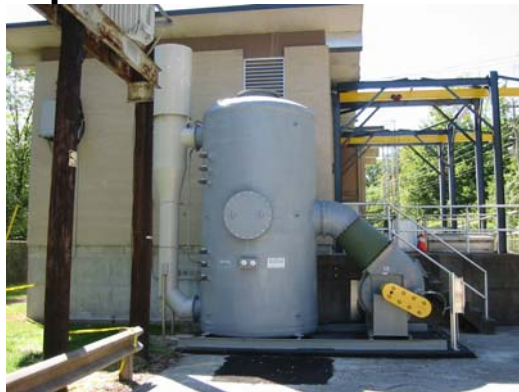
Typical Carbon Adsorber System
