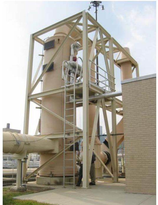
10,500 cfm Primary Clarifier Scrubber
