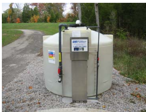
Lakelet Way Chemical Feed System
