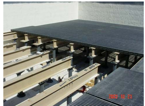
Fiberglass Biofilter Media Support System Inside Lined Tank (No Corrosion)
