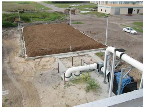
8,300 CFM Screening Structure Biofilter
