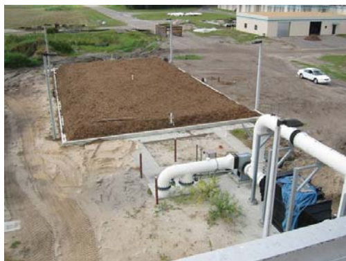
8,300 CFM Screening Structure Biofilter
