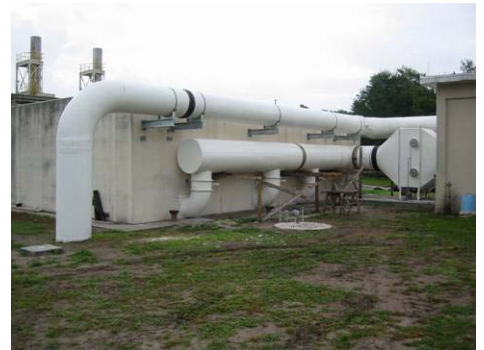
24,000 CFM Biofilter in Existing Sludge Holding Tank
