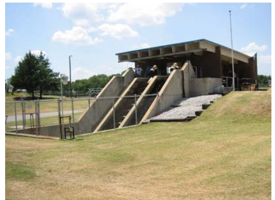
Influent Screw Pumps & Open Headworks
